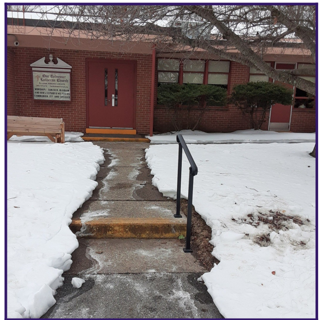
Heavy duty handicap rail has been installed by Bob while kneeling of the frozen ground this winter. Thank you Bob.
